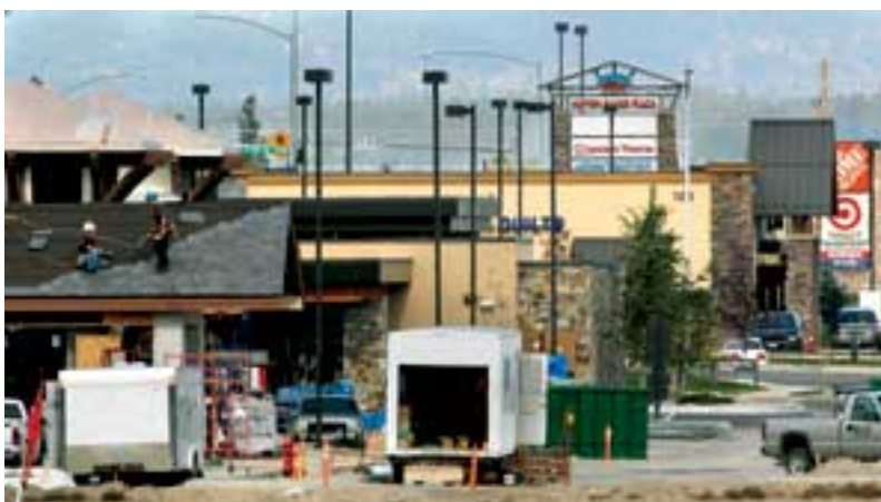
Caption: Construction workers shingle the roof of the Flathead Bank drive-through at Hutton Ranch Plaza in October of 2007. - Lido Vizzutti/Flathead Beacon
